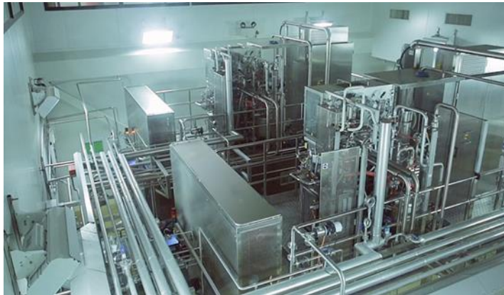
Fonterra's processing line protected by PCS100 AVC
