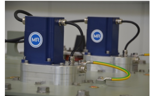
OLTCs top side of the VSR
